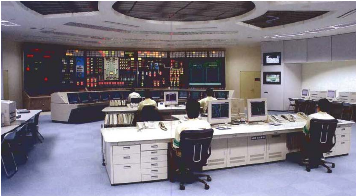
Main control room of RWF
